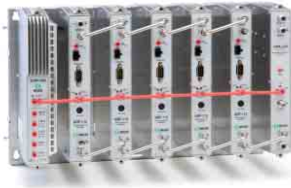
Wall fixing ClassA Headend
