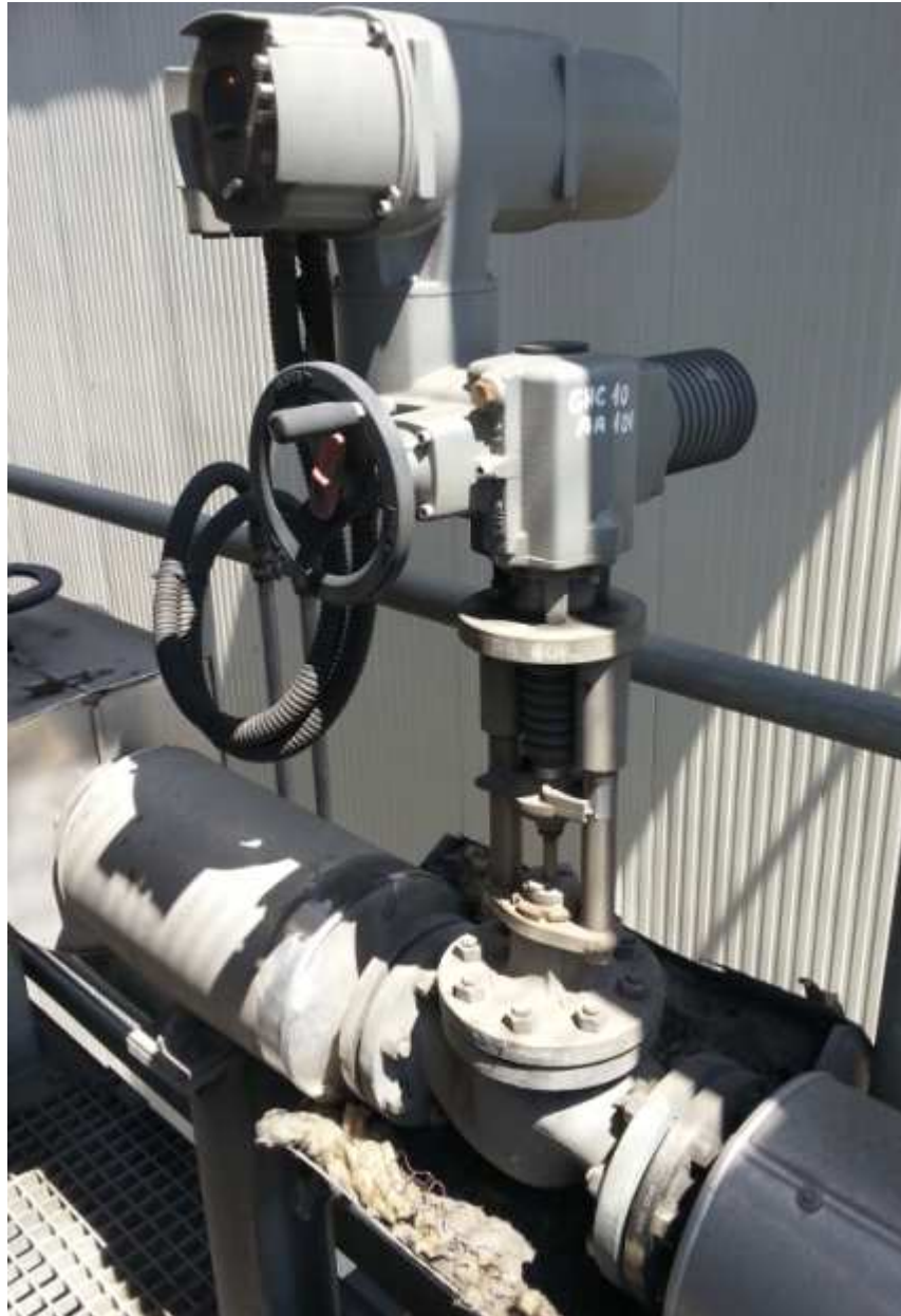
“RTK” Make up water on/off valve
